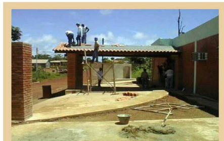
Health Centre, in Bolivar State Venezuela - constructed through a tri-sector partnership between the mining company (Placer Dome and CVG), regional government, local communities, NGOs and the army.
